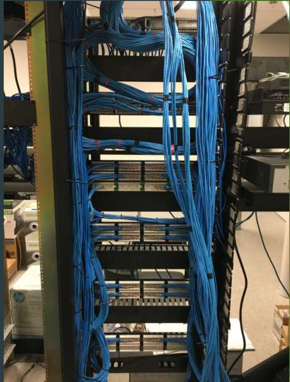
Clean crisp punchdowns, with wiring that is managed correctly
